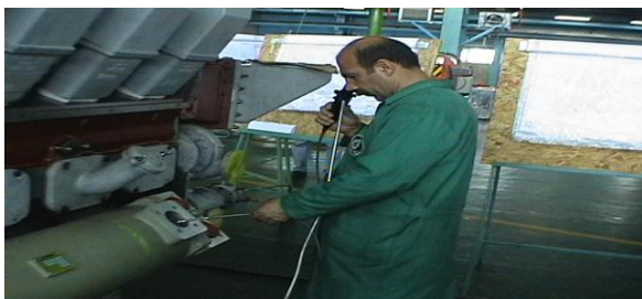
Continuous presence of quality control inspectors to ensure high quality assembly and test procedures
